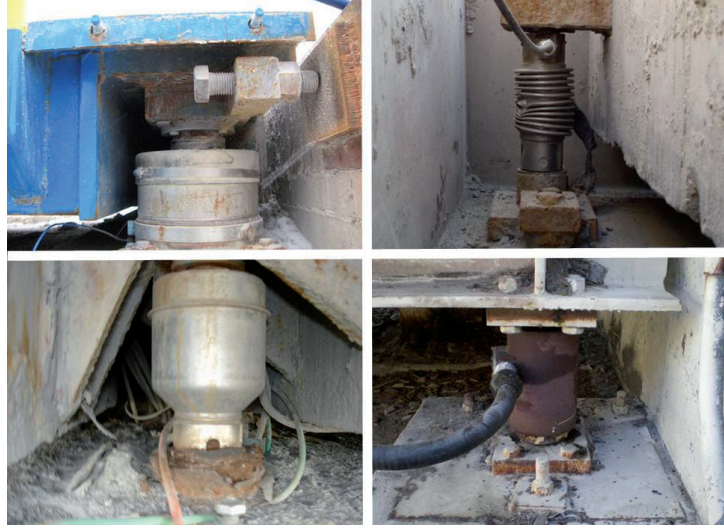
Outdated and vulnerable load cell systems can be the cause of many reoccurring vehicle scale problems.
